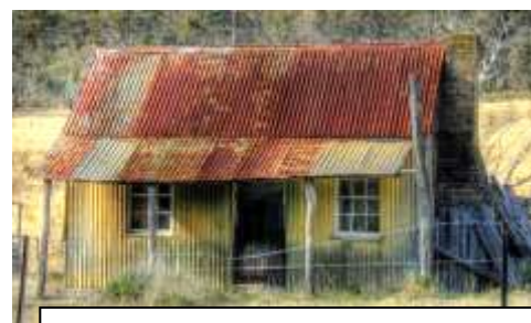
Possibly one of these iron buildings still standing on the road to Mudgee...
